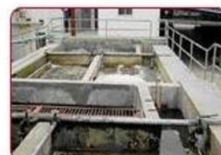
Sewage tank water level measurement
